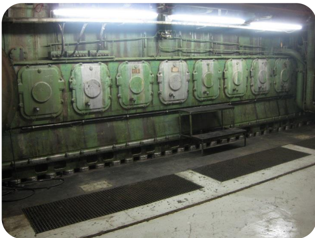
Overview of engine mounted on SKF Vibracon chocks on a concrete foundation.
