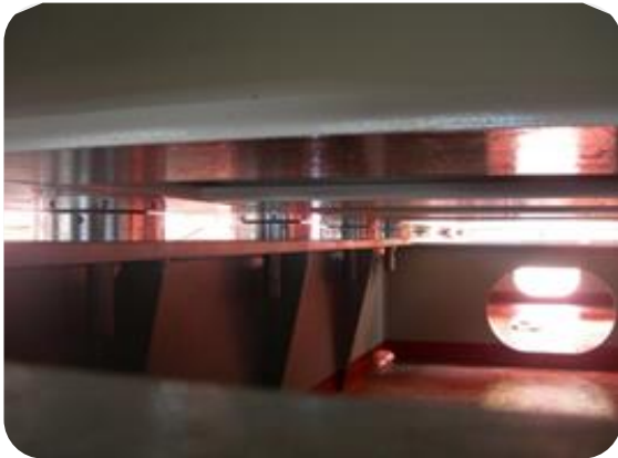
Compressor set chocked and mounted
